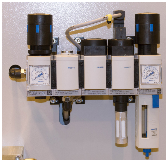
Compressed air connection and regulator
